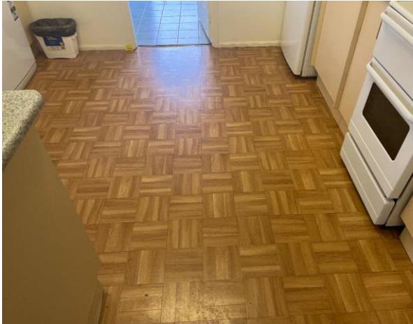
Line ID 18: Internal, Residence, Kitchen, Floor Covering, Timber Look Vinyl Sheet - No Asbestos Detected
