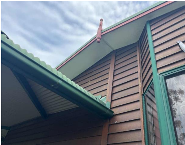
Line ID 3: External, Residence, Throughout, House and Garage, Eaves, Fibre Cement Sheet - No Asbestos Detected
