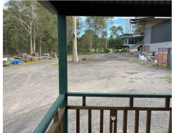
Line ID 24: External, Residence, Throughout, Handrails and Columns, Green Paint - Lead Detected (0.02% w/w)
