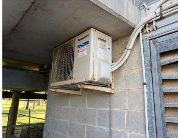
Line ID 42: External, Michael Diamond Building, West Side, on Wall, Panasonic AC Unit, R410A Hydrofluorocarbon (HFC) - Non ODS Refrigerant
