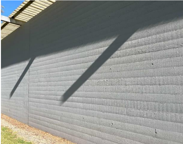
Line ID 23: External, Michael Diamond Building, Throughout, Walls, Grey (Light) Paint - Lead Detected (0.009% w/w)
