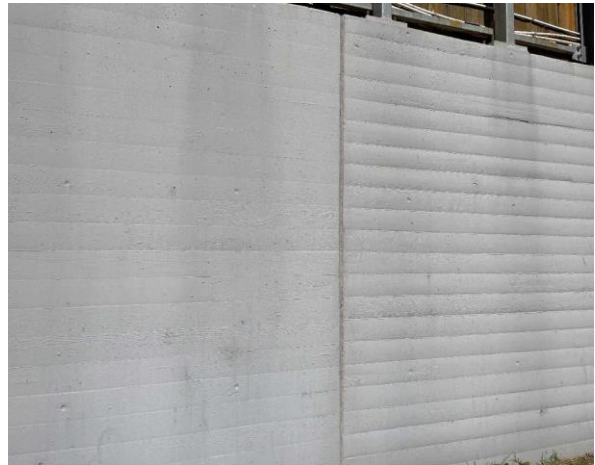
Line ID 2: External, Michael Diamond Building, Throughout, Walls, Expansion Joints, Mastic - No Asbestos Detected
