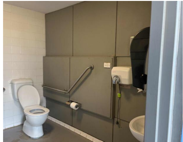
Line ID 20.1: Internal, Russel Mark Control Room, Bathrooms, Male and Disabled Toilet, Wall Panels, Fibre Cement Sheet - No Asbestos Detected
