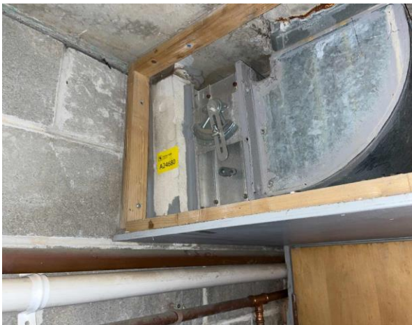
Line ID 16: Internal, Michael Diamond Building, Throughout, Fire Stopping to Ventilation System, Millboard Insulation - No Asbestos Detected
