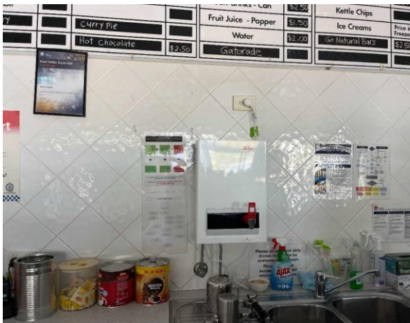
Line ID 31: Internal, Michael Diamond Building, Level 3 Canteen, Above Sink, Hot Water Heater, Insulation Material - Suspected SMF
