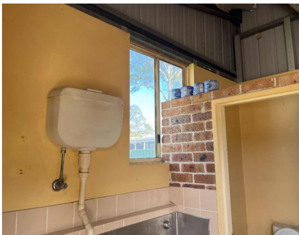
Line ID 5: Internal, Maintenance Shed, Bathroom, Walls, Fibre Cement Sheet - No Asbestos Detected
