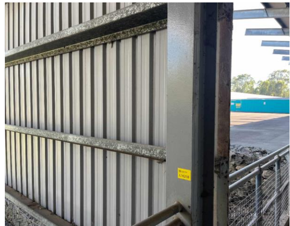
Line ID 22: External, Michael Diamond Building, Throughout, Metal Beams, Grey (Light) Paint - Lead Detected (<0.005% w/w)
