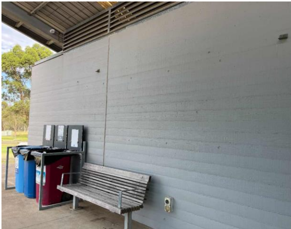
Line ID 25: External, Russell Mark Control Room, Throughout, Walls, Grey Paint - Lead Detected (0.007% w/w)
