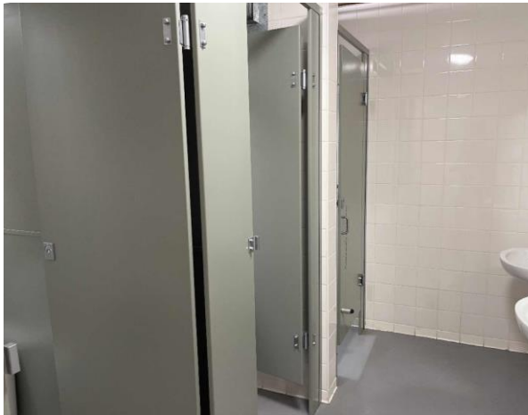
Line ID 7: Internal, Michael Diamond Building, Level 1, Toilets, Partition Walls, Fibre Cement Sheeting - No Asbestos Detected
