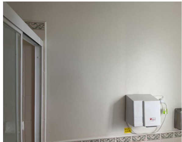
Line ID 17: Internal, Residence, Bathrooms, Walls, Fibre Cement Sheet - No Asbestos Detected
