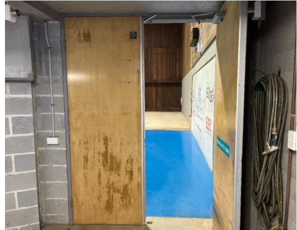
Line ID 15.1: Internal, Michael Diamond Building, Throughout, Fire Door, Fire Door Core - No Asbestos Detected
