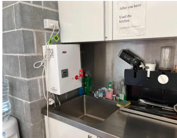
Line ID 38: Internal, Russel Mark Control Room, Kitchen, Above Sink, Hot Water Boiler, Internal Insulation - Suspected SMF
