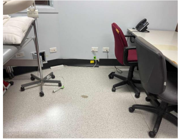
Line ID 14: Internal, Michael Diamond Building, Percy Pavey Range, First Aid Office, Skirting Board, Black Vinyl - No Asbestos Detected
