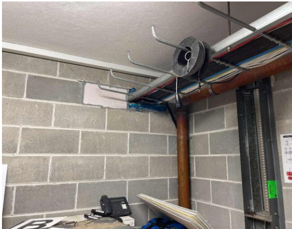
Line ID 36.1: Internal, Michael Diamond Building, Throughout, Penetrations, Pillow Insulation - Suspected SMF
