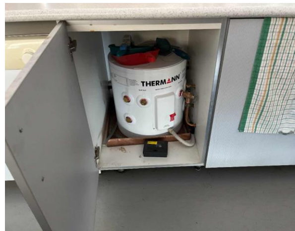
Line ID 32: Internal, Michael Diamond Building, Level 3 Canteen, Under Sink, Hot Water Heater, Insulation Material - Suspected SMF
