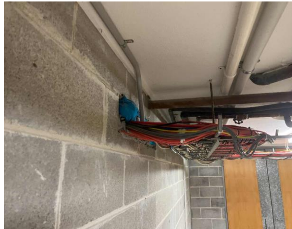
Line ID 36: Internal, Michael Diamond Building, Throughout, Penetrations, Pillow Insulation - Suspected SMF
