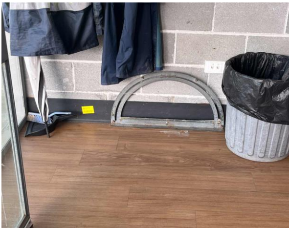
Line ID 21: Internal, Russel Mark Control Room, Bathrooms, Office and Kitchen, Skirting, Black Vinyl Skirting - No Asbestos Detected
