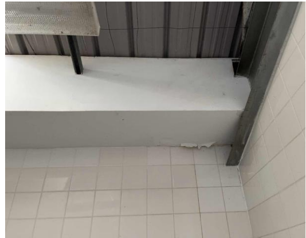
Line ID 26: Internal, Russel Mark Control Room, Bathrooms, High Level Boxing, White Paint - Lead Detected (<0.005% w/w)
