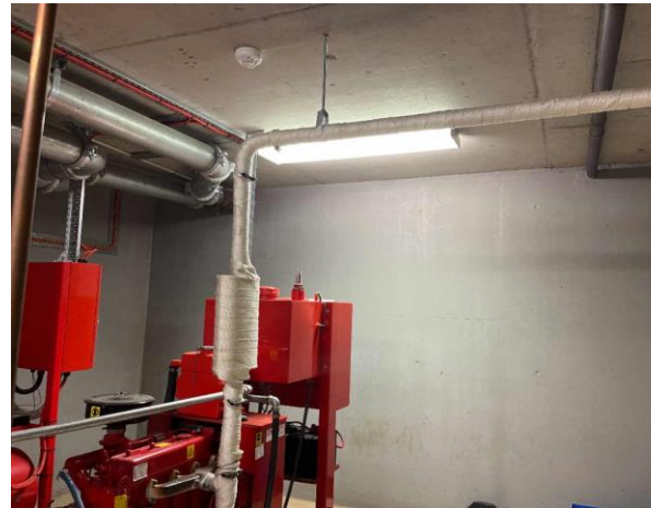
Line ID 30: Internal, Michael Diamond Building, Level 2 Fire Hydrant Room, Diesel Fire Pump Pipework, Insulation Material - Suspected SMF
