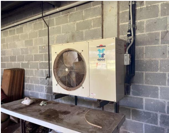
Line ID 43: External, Michael Diamond Building, West Side, SunDowner AC Unit, Unknown Refrigerant - Suspected ODS
