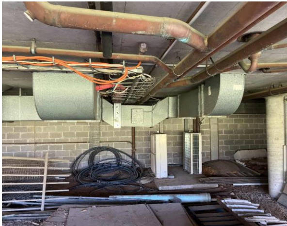
Line ID 1: External, Michael Diamond Building, Throughout, Ductwork, Electrical Distribution Heater, Millboard Insulation - Suspected Asbestos
