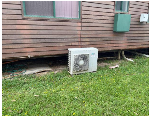
Line ID 44: External, Residence, North East Side, Daikin AC Unit, R410A Hydrofluorocarbon (HFC) - Non ODS Refrigerant
