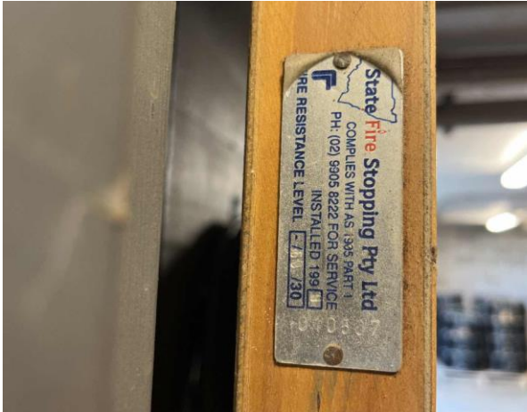
Line ID 15: Internal, Michael Diamond Building, Throughout, Fire Door, Fire Door Core - No Asbestos Detected
