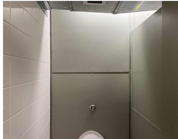
Line ID 8: Internal, Michael Diamond Building, Level 1, Walls Behind Toilets, Fibre Cement Sheet - No Asbestos Detected
