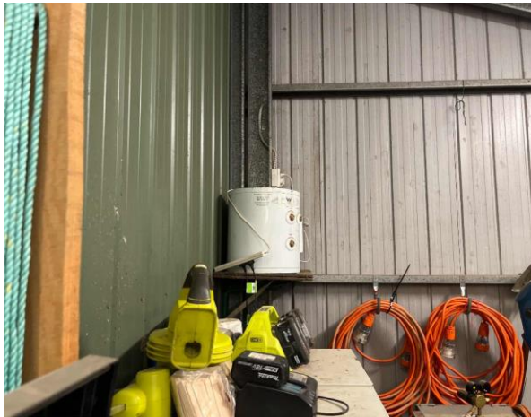
Line ID 29: Internal, Maintenance Shed, Cage Area, Hot Water Heater, Insulation Material - Suspected SMF
