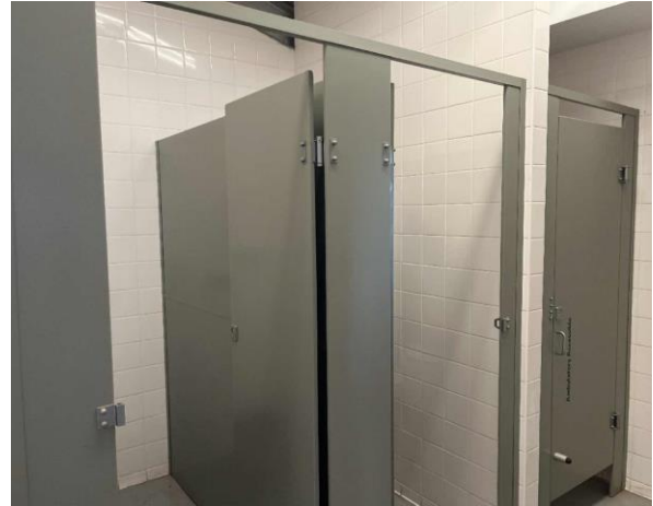
Line ID 19: Internal, Russel Mark Control Room, Bathrooms, Cubicle Partition Walls, Compressed Cement Sheet - No Asbestos Detected
