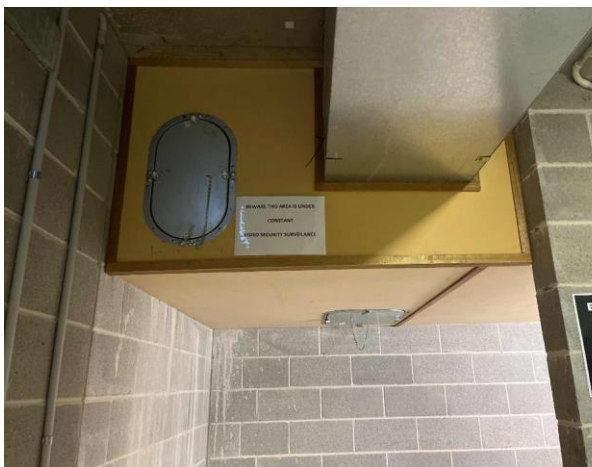
Line ID 33: Internal, Michael Diamond Building, Throughout, Air Conditioning Ductwork, Internal Insulation - Suspected SMF
