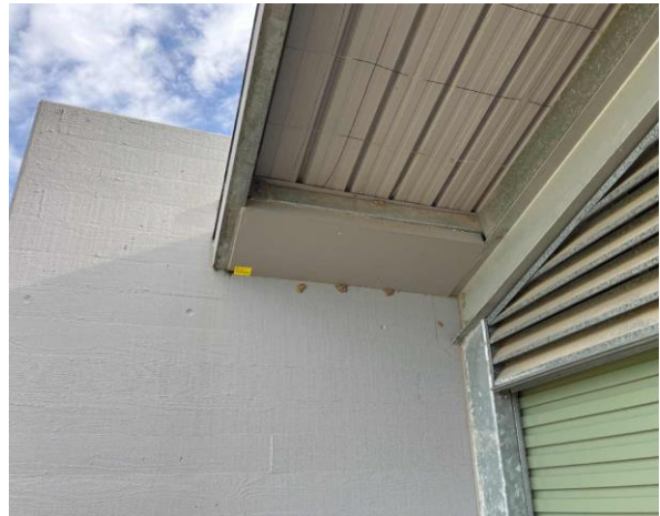
Line ID 4: External, Russell Mark Control Room, West Side, High Level Boxing, Fibre Cement Sheet - No Asbestos Detected
