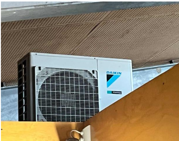
Line ID 45: Internal, Michael Diamond Building, Level 3, Above Offices, R410A Hydrofluorocarbon (HFC) - Non ODS Refrigerant
