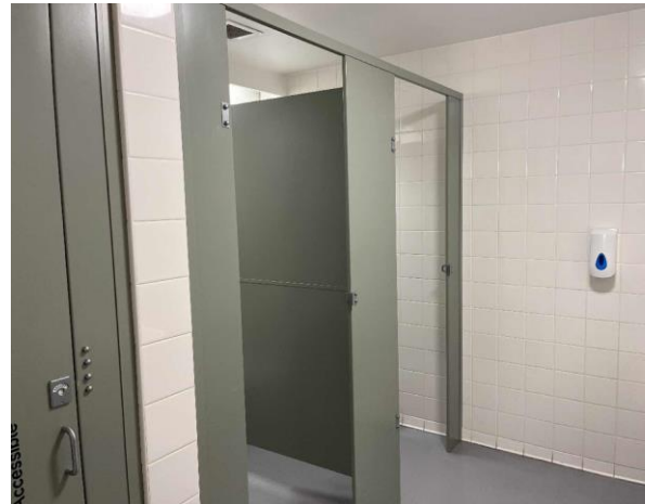
Line ID 10: Internal, Michael Diamond Building, Level 2, Toilets, Partition Walls, Fibre Cement Sheeting - No Asbestos Detected
