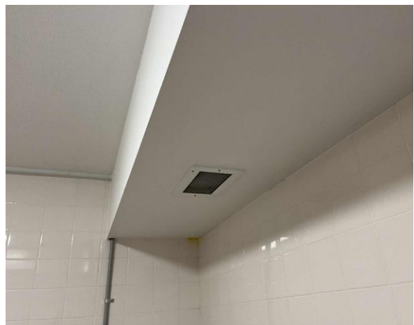
Line ID 6: Internal, Michael Diamond Building, Level 1, Bathrooms, Boxing to Ventilation System, Fibre Cement Sheet - No Asbestos Detected
