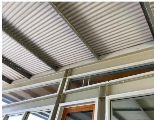
Line ID 21.1: Internal, Boatsheds, Throughout, L1, Fascia and Walls, Fibre Cement Sheeting - No Asbestos Detected
