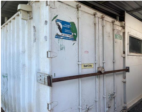
Line ID 77: External, Old Compound, Throughout, Shipping Container Walls, White Paint - Lead Detected (0.36% w/w)
