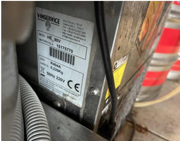
Line ID 117.1: Internal, Restaurant, West Dining Room, Bar Area, Under Bench Chiller, R404a Refrigerant - Non ODS Refrigerant
