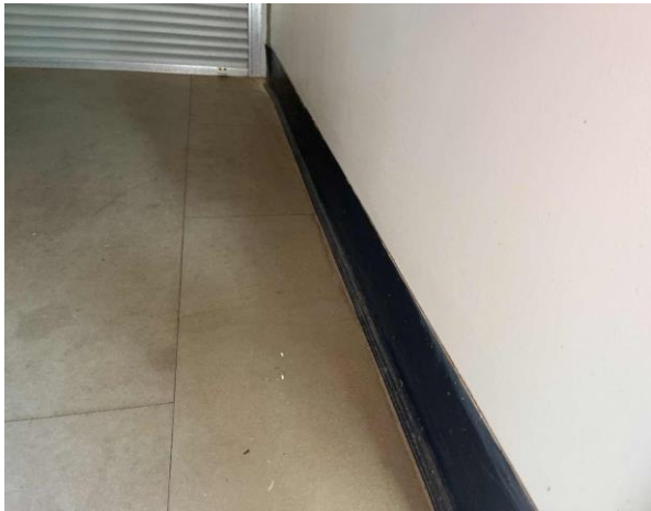
Line ID 70: Internal, Timing Towers, Tower at 500m, Skirting, Black Vinyl Sheet - No Asbestos Detected
