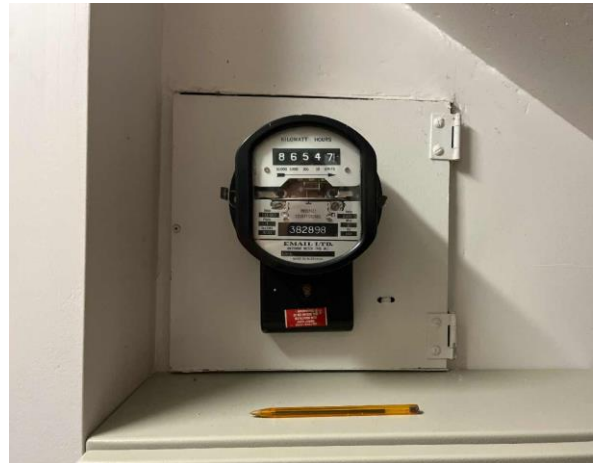
Line ID 29: Internal, Finish Tower, GF, Electrical and MDF Room, Electrical Meter, Mastic and Glazing - Suspected Asbestos
