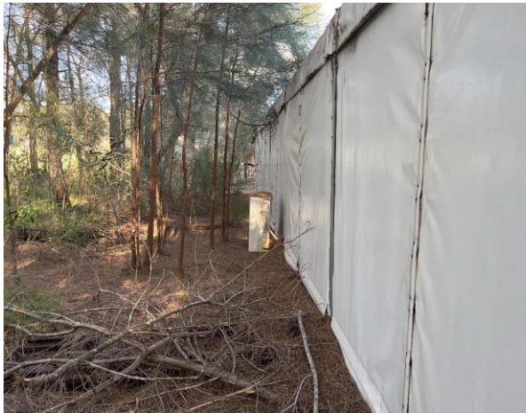
Line ID 110: External, Old Compound, South East Side, AC Unit, R22 Hydrochlorofluorocarbon (HCFC) - ODS Refrigerant
