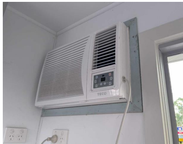
Line ID 115: Internal, Front Gate Security Office, Throughout, TECO AC Unit, Unknown Refrigerant - Suspected ODS
