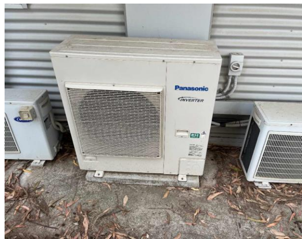
Line ID 112: External, Venue Operations Centre, South Side of Building, Panasonic AC Unit, R32 Refrigerant - Non ODS Refrigerant
