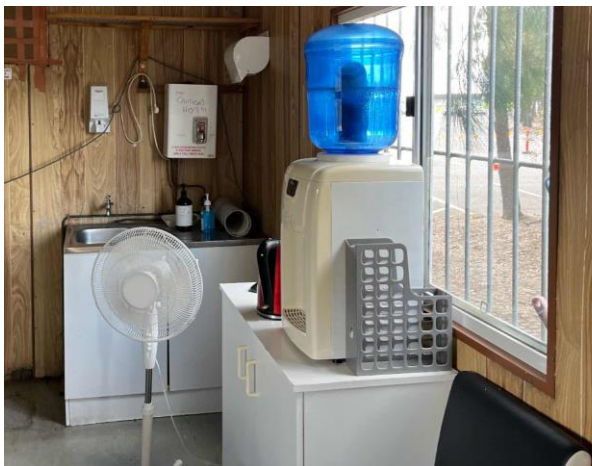
Line ID 114.1: Internal, Cleaners Office, Kitchenette, Water Cooler, R32 Hydrofluorocarbon (HFC) - Non ODS Refrigerant
