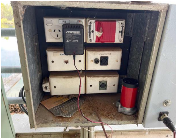
Line ID 3: External, Finish Tower, L3, Balcony, Switchboard, Bituminous Backing Board - No Asbestos Suspected
