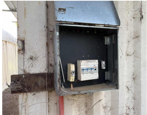
Line ID 9: External, Old Compound, North Building, South Corner, Switchboard, Bituminous Backing Board - No Asbestos Suspected
