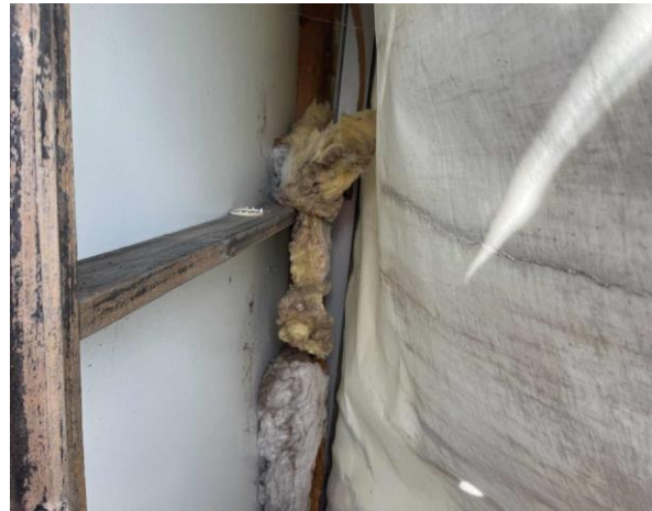
Line ID 83: External, Old Compound, Throughout, Behind Walls, Insulation Batts - Suspected SMF
