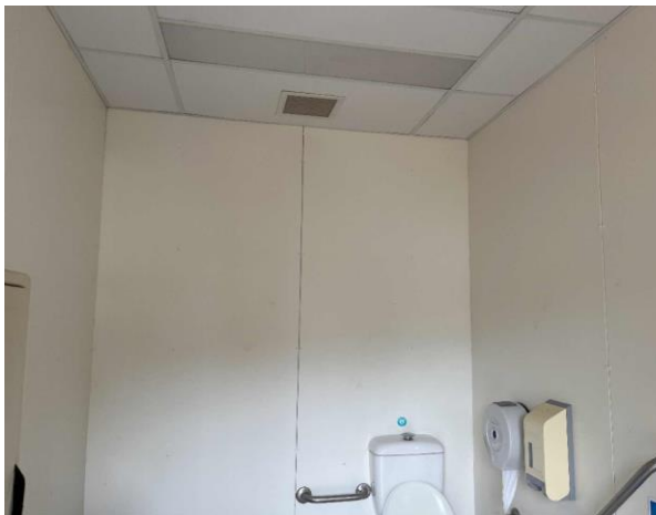
Line ID 42: Internal, Restaurant, North Externally Accessed Toilets, Walls, Fibre Cement Sheeting - No Asbestos Detected
