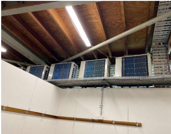
Line ID 113: Internal, Boatsheds, Female Toilets, North Wall, AC Units, R410A Hydrofluorocarbon (HFC) - Non ODS Refrigerant
