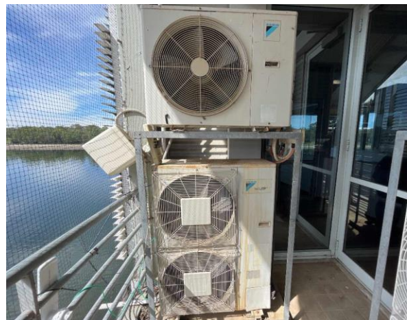
Line ID 106: External, Finish Tower, L2, Balcony, Daikin AC Units, R22 Hydrochlorofluorocarbon (HCFC) - ODS Refrigerant
