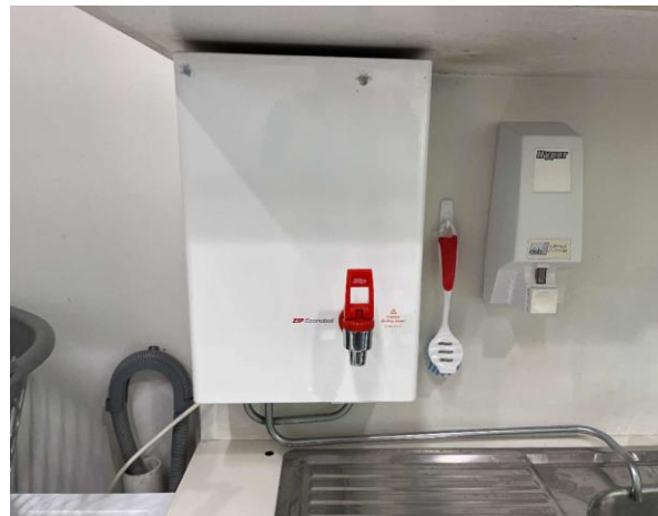
Line ID 98: Internal, Venue Operations Centre, Kitchen, Boiler, Internal Insulation - Suspected SMF
