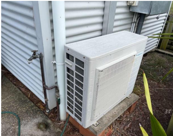
Line ID 108: External, First Aid Building, East Side, Daikin AC unit, R410A Hydrofluorocarbon (HFC) - Non ODS Refrigerant
