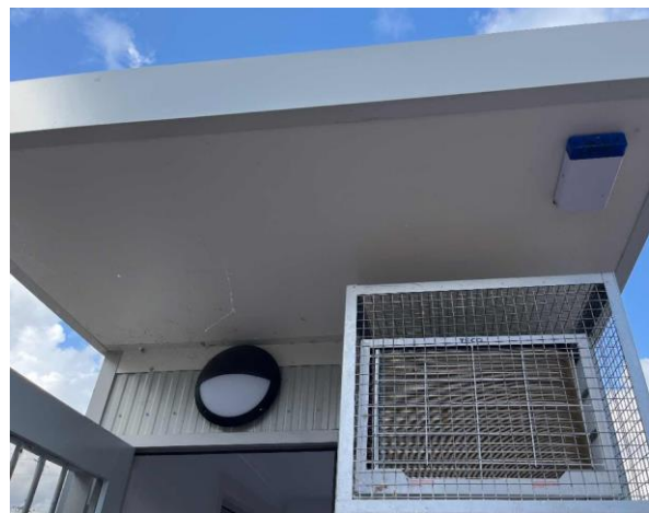
Line ID 6: External, Front Gate Security Office, Throughout, Eaves, Fibre Cement Sheet - No Asbestos Detected
