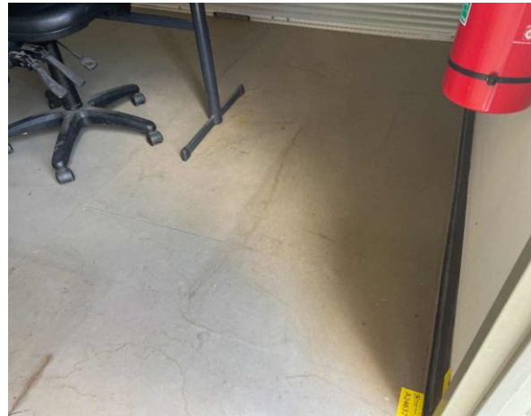
Line ID 65: Internal, Timing Towers, Tower at 1750m, Floor Lining, Fibre Cement Sheet - No Asbestos Detected
