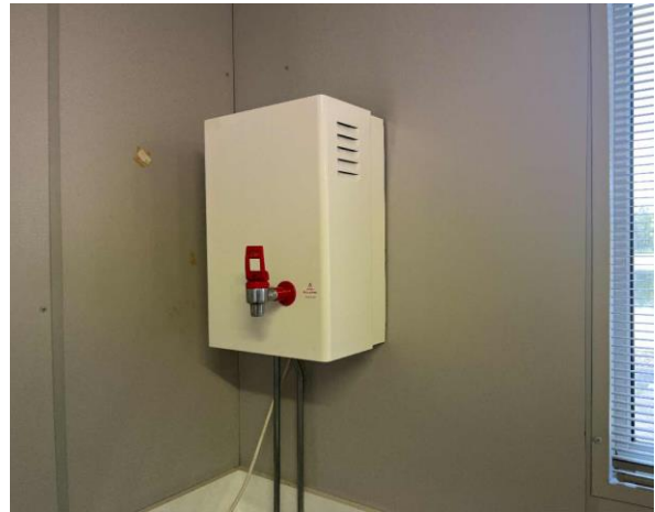
Line ID 90: Internal, First Aid Building, Throughout, Hot Water Boiler, Internal Insulation - Suspected SMF
