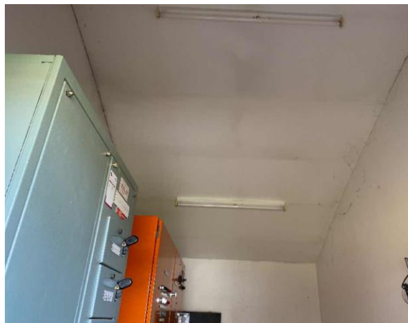
Line ID 25: Internal, Communications Building, Throughout, Main Switch Room, Ceiling, Fibre Cement Sheet - No Asbestos Detected
