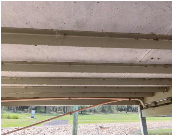
Line ID 52: Internal, Timing Towers, Tower at 0m, Floor, Fibre Cement Sheet - No Asbestos Detected
