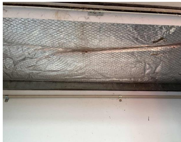
Line ID 100: Internal, Venue Operations Centre, Throughout, Ceiling, Sarking Insulation - Suspected SMF
