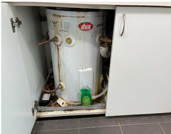
Line ID 99: Internal, Venue Operations Centre, Kitchen, Hot Water Heater, Insulation Material - Suspected SMF
