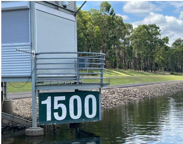
Line ID 14: External, Timing Towers, Tower at 1500m, Switchboard, Bituminous Backing Board - No Asbestos Suspected
