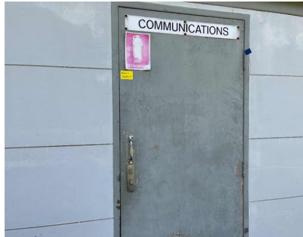
Line ID 76: External, Communications Shed, Throughout, Doors, Green Paint - Lead Detected (0.007% w/w)
