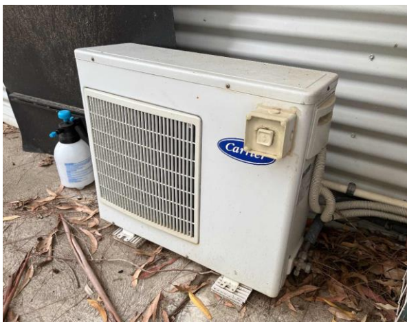
Line ID 111.1: External, Venue Operations Centre, South Side of Building, Carrier AC Unit, R22 Hydrochlorofluorocarbon (HCFC) - ODS Refrigerant
