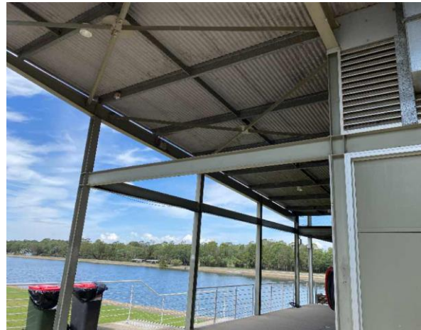
Line ID 78: External, Restaurant, Throughout, Steelwork, Green Paint - Lead Detected (<0.005% w/w)
