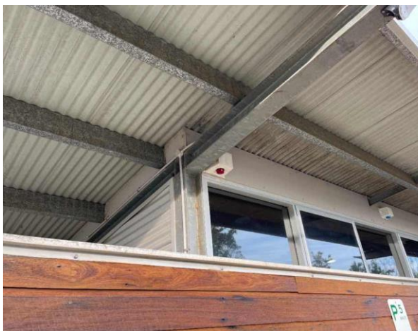
Line ID 16: External, Venue Operations Centre, Throughout, Fascia, Fibre Cement Sheet - No Asbestos Detected
