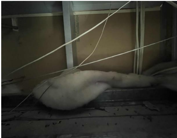
Line ID 101: Internal, Venue Operations Centre, Throughout, Ceiling Space, Insulation Batts - Suspected SMF
