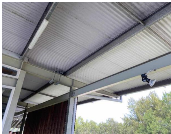
Line ID 74.1: External, Boatsheds, Throughout, Veranda, Steelwork and Railings, Green Paint - Lead Detected (0.058% w/w)
