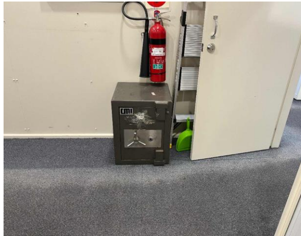
Line ID 22: Internal, Boatsheds, Venue Management Office, Within Safe, Internal Insulation - Suspected Asbestos
