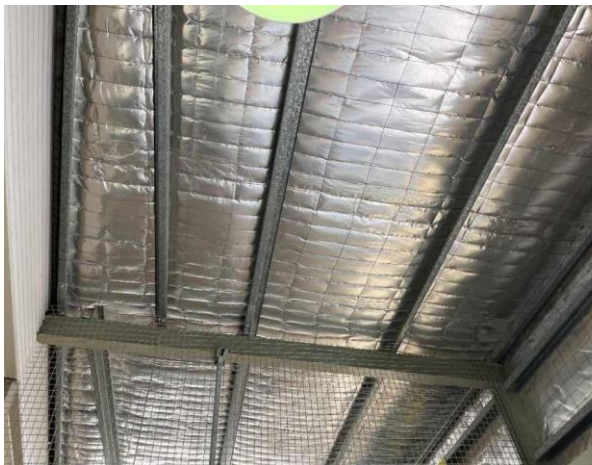
Line ID 84: Internal, Boatsheds, Throughout, Ceiling, Sarking Insulation - Suspected SMF
