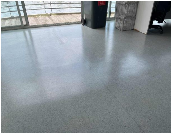
Line ID 28: Internal, Finish Tower, GF, Floor Covering, Blue Speckled Vinyl Sheet - No Asbestos Detected
