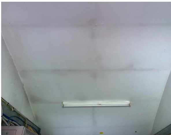
Line ID 24: Internal, Communications Building, Throughout, Ceiling, Fibre Cement Sheet - No Asbestos Detected
