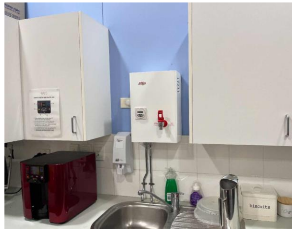
Line ID 85: Internal, Boatsheds, Venue Management Office, Hot Water Boiler, Internal Insulation - Suspected SMF
