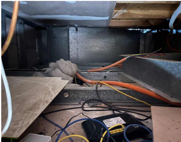
Line ID 82: Internal, Restaurant, Kitchen, Ceiling Space, Dust - Lead Detected (35 mg/kg)
