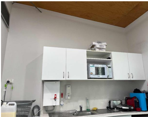
Line ID 72: Internal, Venue Operations Centre, Kitchen, Wall Behind Sink, Fibre Cement Sheet - No Asbestos Detected
