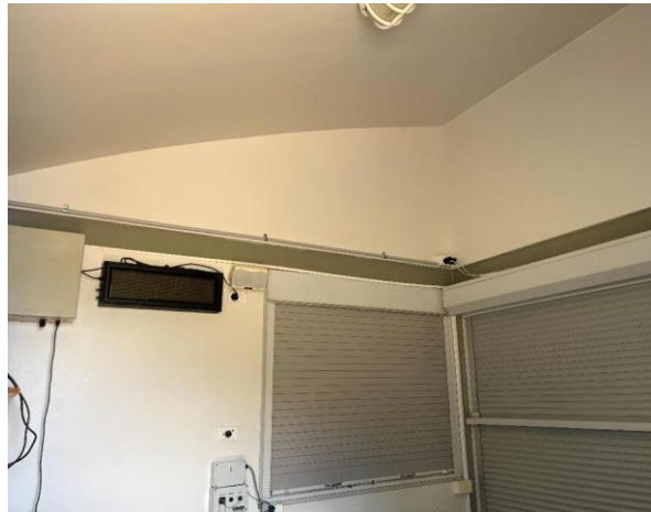
Line ID 71: Internal, Timing Towers, Tower at 500m, Walls and Ceiling, Fibre Cement Sheet - No Asbestos Detected
