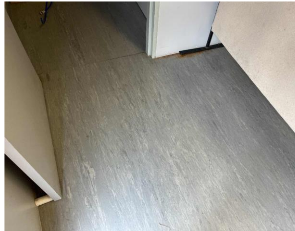
Line ID 35: Internal, First Aid Building, Throughout, Floor Covering, Blue Vinyl Sheet - No Asbestos Detected
