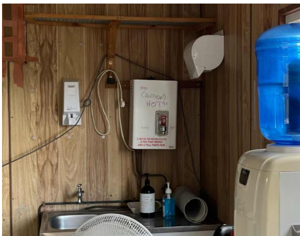
Line ID 86: Internal, Cleaners Office, Kitchenette, Above Sink, Hot Water Boiler, Internal Insulation - Suspected SMF
