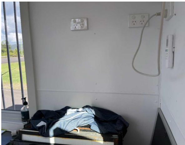
Line ID 36: Internal, Front Gate Security Office, Throughout, Walls, Fibre Cement Sheet - No Asbestos Detected
