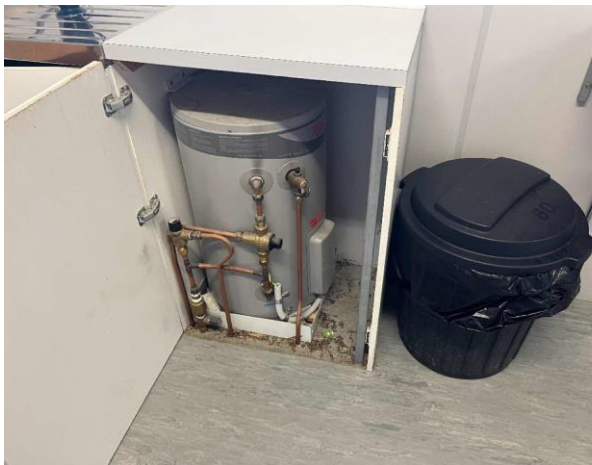
Line ID 91: Internal, First Aid Building, Throughout, Under Sink, Hot Water Heater, Internal Insulation - Suspected SMF
