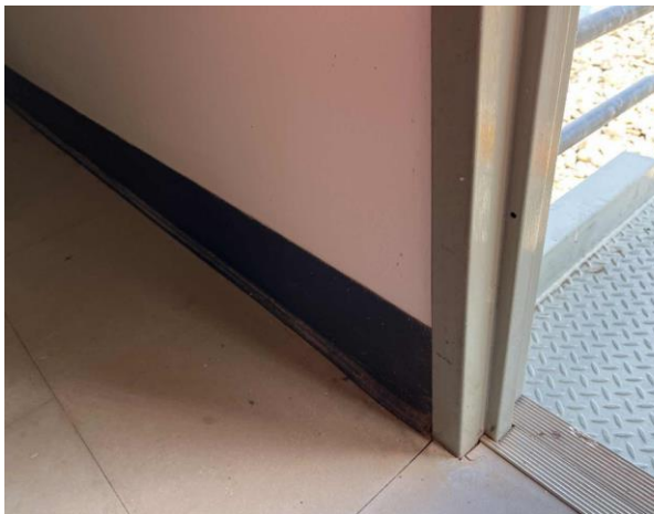
Line ID 54: Internal, Timing Towers, Tower at 0m, Skirting, Black Vinyl Sheet - No Asbestos Detected
