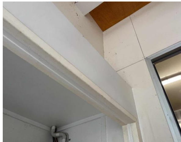
Line ID 43: Internal, Restaurant, North Storage Area, Walls, Fibre Cement Sheeting - No Asbestos Detected
