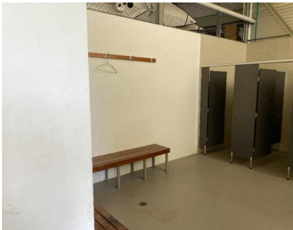
Line ID 19: Internal, Boatsheds, Male Toilets, Walls, Fibre Cement Sheeting - No Asbestos Detected
