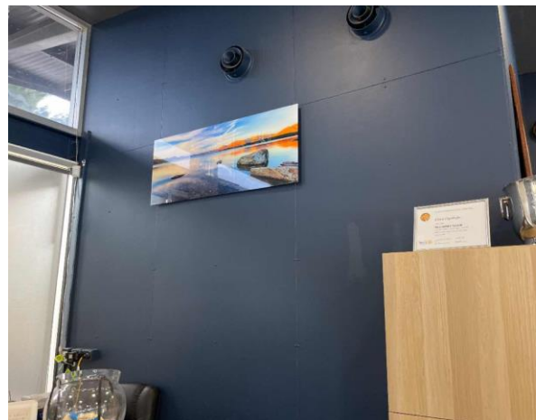
Line ID 45: Internal, Restaurant, West Dining Room, Walls, Fibre Cement Sheeting - No Asbestos Detected
