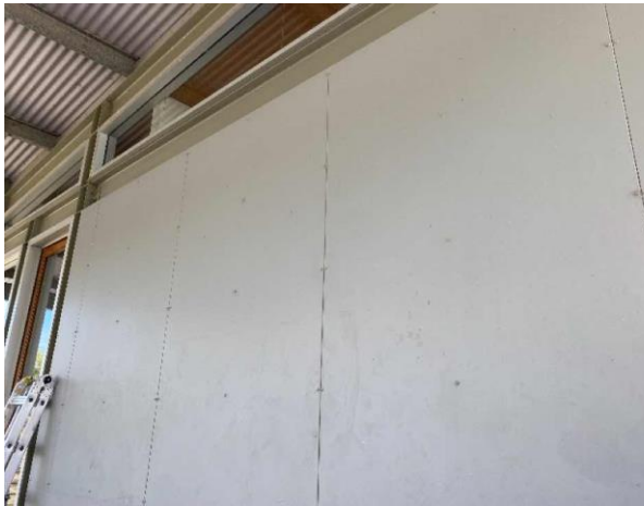
Line ID 21.2: Internal, Boatsheds, Throughout, L1, Fascia and Walls, Fibre Cement Sheetting - No Asbestos Detected
