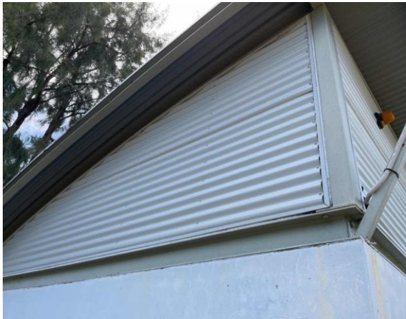
Line ID 75: External, Communications Shed, Throughout, Beams, Green Paint - Lead Detected (<0.005% w/w)
