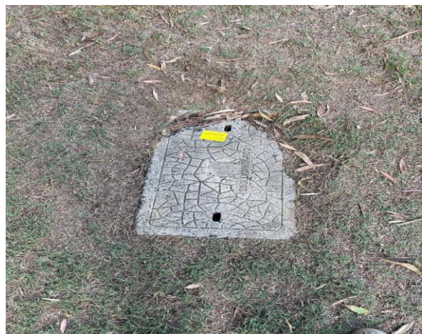
Line ID 5: External, First Aid Building, West Grass Area, Comms Pit, Compressed Cement - No Asbestos Detected
