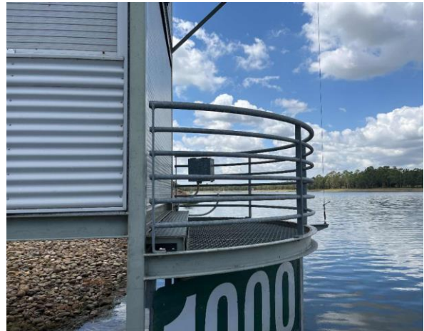
Line ID 13: External, Timing Towers, Tower at 1000m, Switchboard, Bituminous Backing Board - No Asbestos Suspected
