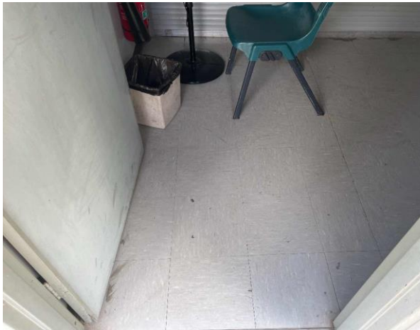
Line ID 48: Internal, Start Line Tower, Throughout, Floor Covering, Light Blue Vinyl Tiles - No Asbestos Detected
