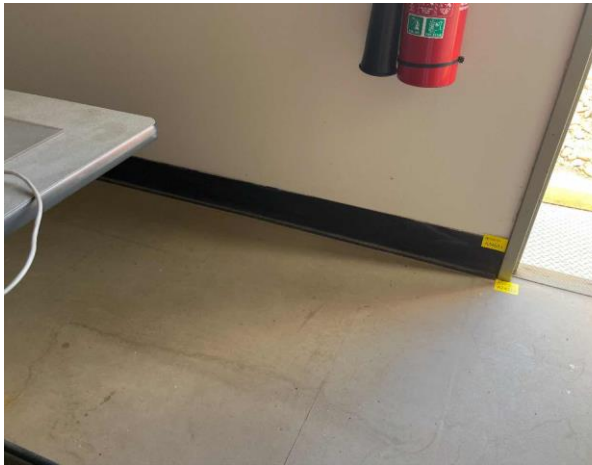
Line ID 66: Internal, Timing Towers, Tower at 1750m, Skirting Boards, Black Vinyl Sheet - No Asbestos Detected
