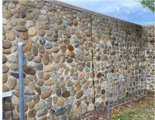
Line ID 7.1: External, Grounds, Entrance Wall, Expansion Gap, Bituminous Membrane - No Asbestos Detected
