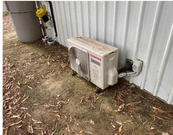
Line ID 109: External, Maintenance Shed, Throughout, North Elevation, AC Unit, R410A Hydrofluorocarbon (HFC) - Non ODS Refrigerant
