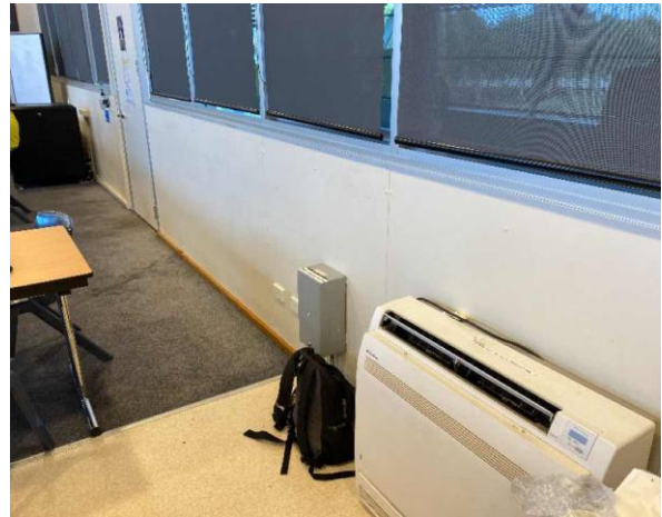
Line ID 18: Internal, Boatsheds, L1, Offices, Walls, Fibre Cement Sheeting - No Asbestos Detected
