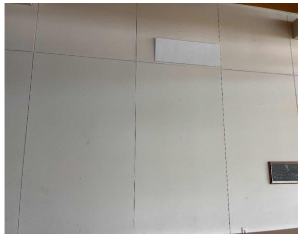
Line ID 39: Internal, Restaurant, East Dining Room, Walls, Fibre Cement Sheet - No Asbestos Detected
