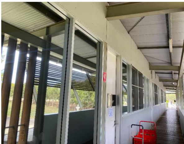
Line ID 21: Internal, Boatsheds, Throughout, L1, Fascia and Walls, Fibre Cement Sheeting - No Asbestos Detected
