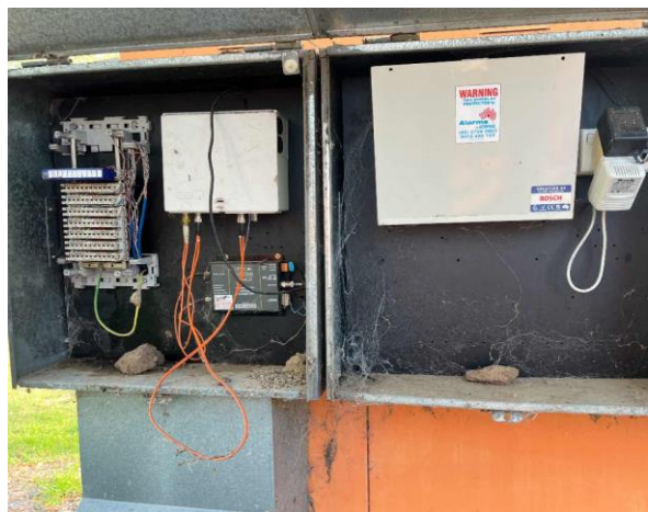
Line ID 27: Internal, Electrical Kiosk adj Gate B, South Side, Switchboard, Bituminous Backing Board - No Asbestos Suspected
