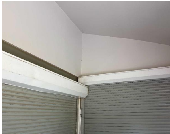
Line ID 51: Internal, Start Line Tower, Throughout, Walls and Ceiling, Fibre Cement Sheet - No Asbestos Detected
