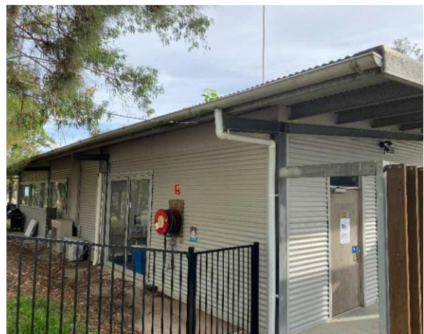
Line ID 16.1: External, Venue Operations Centre, Throughout, Fascia, Fibre Cement Sheet - No Asbestos Detected
