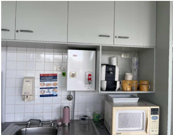
Line ID 89: Internal, Finish Tower, GF, Entrance Hallway, Zip Boiler, Internal Insulation - Suspected SMF
