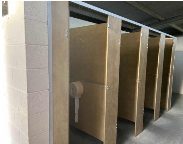
Line ID 47: Internal, South West Toilet Block, Toilets, Cubicle Partition Wall, Fibre Cement Sheet - No Asbestos Detected
