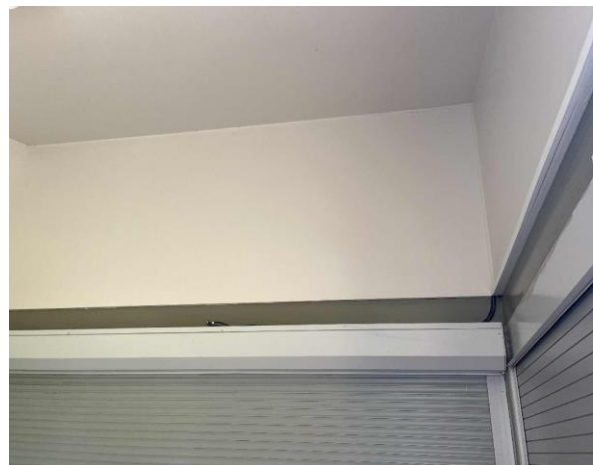
Line ID 63: Internal, Timing Towers, Tower at 1500m, Walls and Ceiling, Fibre Cement Sheet - No Asbestos Detected
