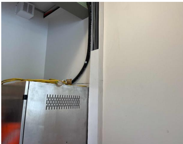
Line ID 30: Internal, Finish Tower, GF, Electrical and MDF Room, Walls, Fibre Cement Sheet - No Asbestos Detected
