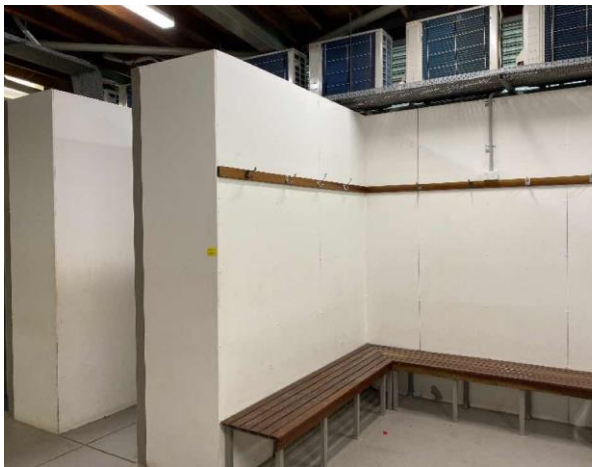
Line ID 79: Internal, Boatsheds, Female Toilets, Walls, White Paint - Lead Detected (<0.005% w/w)
