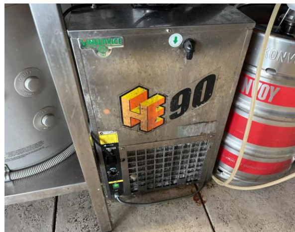
Line ID 117: Internal, Restaurant, West Dining Room, Bar Area, Under Bench Chiller, R404a Refrigerant - Non ODS Refrigerant
