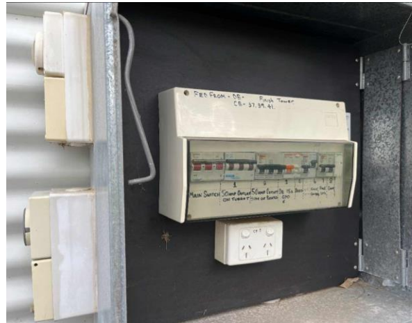
Line ID 4: External, First Aid Building, East Side, Switchboard, Bituminous Backing Board - No Asbestos Suspected
