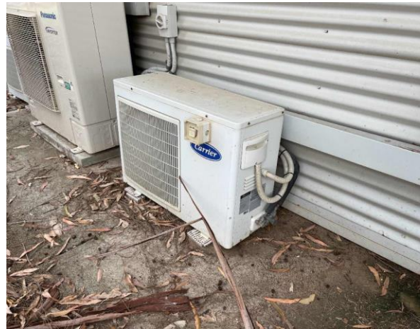
Line ID 111: External, Venue Operations Centre, South Side of Building, Carrier AC Unit, R22 Hydrochlorofluorocarbon (HCFC) - ODS Refrigerant
