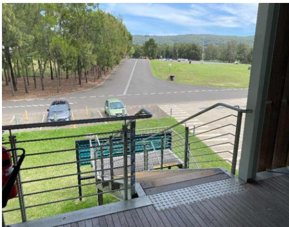
Line ID 74: External, Boatsheds, Throughout, Veranda, Steelwork and Railings, Green Paint - Lead Detected (0.058% w/w)
