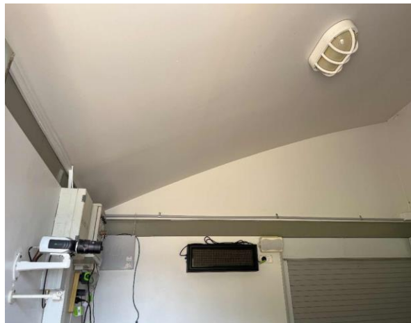
Line ID 55: Internal, Timing Towers, Tower at 0m, Walls and Ceiling, Fibre Cement Sheet - No Asbestos Detected
