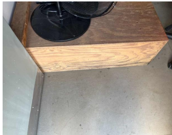
Line ID 69: Internal, Timing Towers, Tower at 500m, Floor Lining below Vinyl, Fibre Cement Sheet - No Asbestos Detected
