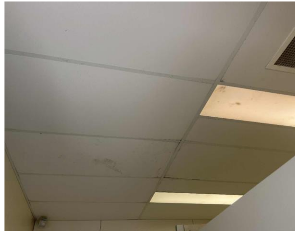
Line ID 96: Internal, Restaurant, North Externally Accessed Toilets, Ceiling, Compressed Ceiling Tiles - Suspected SMF
