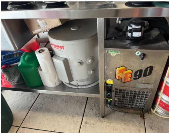
Line ID 97: Internal, Restaurant, West Dining Room, Bar Area Under Sink, Hot Water Heater, Internal Insulation - Suspected SMF
