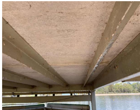
Line ID 61: Internal, Timing Towers, Tower at 1500m, Floor Lining below Vinyl, Compressed Cement Sheet - No Asbestos Detected
