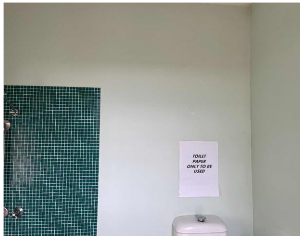
Line ID 73: Internal, Venue Operations Centre, Toilets, Walls, Fibre Cement Sheet - No Asbestos Detected
