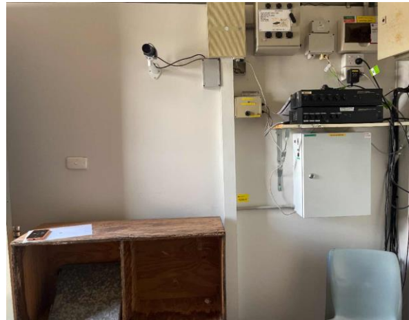
Line ID 67: Internal, Timing Towers, Tower at 1750m, Walls and Ceiling, Fibre Cement Sheet - No Asbestos Detected
