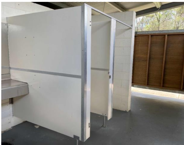
Line ID 38: Internal, North East Toilets, Throughout, Cubicle Partition Walls, Compressed Cement Sheet - No Asbestos Detected
