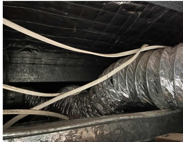
Line ID 102: Internal, Venue Operations Centre, Throughout, Ceiling Space, Flexible Ductwork, Insulation Material - Suspected SMF
