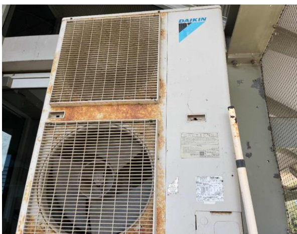
Line ID 106.1: External, Finish Tower, L2, Balcony, Daikin AC Units, R22 Hydrochlorofluorocarbon (HCFC) - ODS Refrigerant
