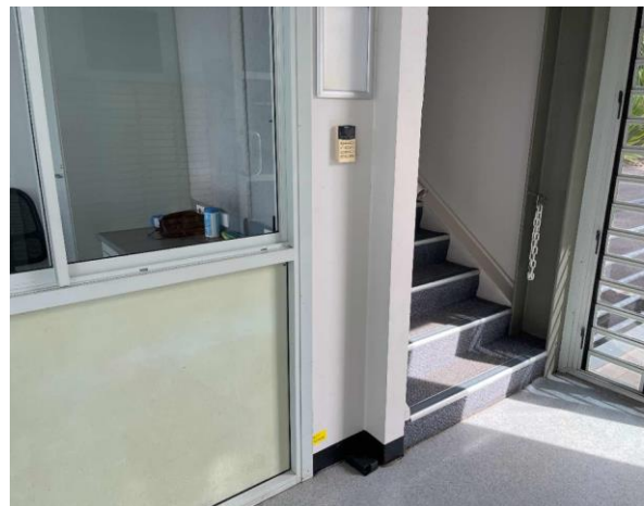
Line ID 31: Internal, Finish Tower, GF, Entrance Hallway, Walls, Fibre Cement Sheet - No Asbestos Detected
