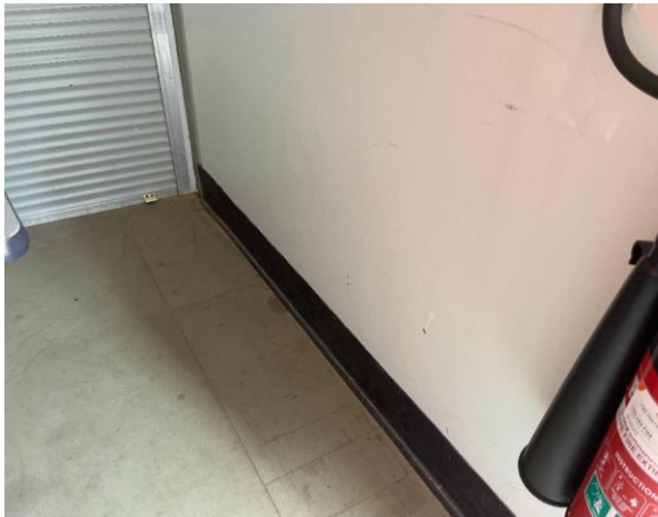
Line ID 58: Internal, Timing Towers, Tower at 1000m, Skirting, Black Vinyl Sheet - No Asbestos Detected
