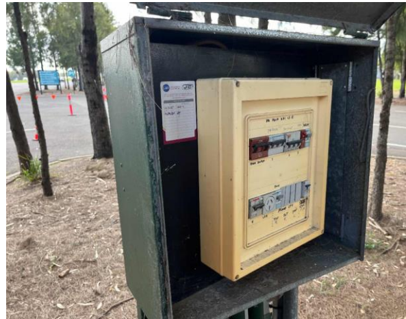
Line ID 2: External, Cleaners Office, South Side, Switchboard, Bituminous Backing Board - No Asbestos Suspected
