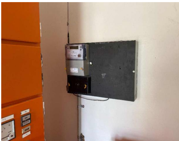
Line ID 26: Internal, Communications Building, Throughout, Switchboard, Bituminous Backing Board - No Asbestos Suspected
