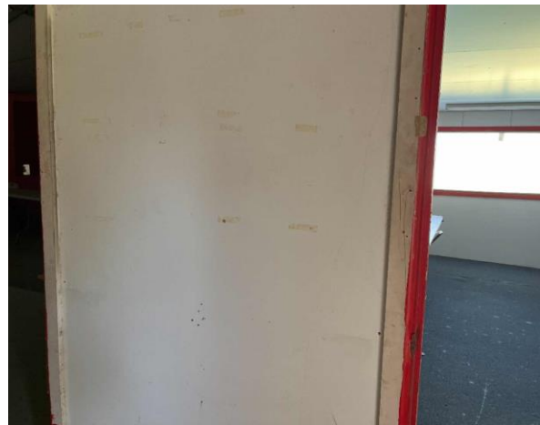
Line ID 81: Internal, Old Compound, Throughout, Walls, White Paint - Lead Detected (<0.005% w/w)
