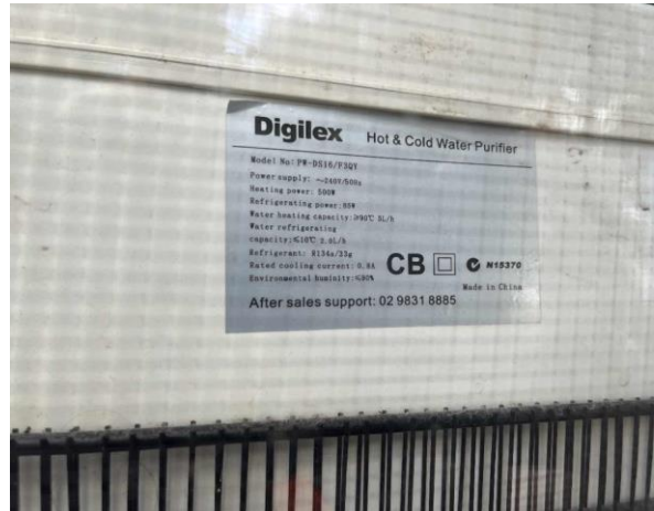
Line ID 114: Internal, Cleaners Office, Kitchenette, Water Cooler, R32 Hydrofluorocarbon (HFC) - Non ODS Refrigerant
