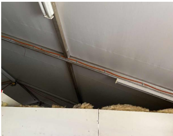
Line ID 93: Internal, Old Compound, Throughout, Above Kitchen, Ceiling, Loose Insulation - Suspected SMF
