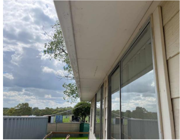
Line ID 12: External, House, Perimeter, Eaves, Fibre Cement Sheet - Chrysotile Asbestos Detected
