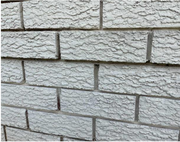
Line ID 11: External, House, Perimeter, Damp Proof Course to Brickwork, Waterproof Membrane - No Asbestos Detected
