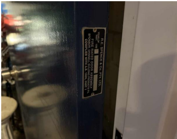
Line ID 32.1: Internal, Main Arena 1, Eastern Storage Area, Door to E.05, E.04 and E.03, Fire Door Core - Suspected Asbestos
