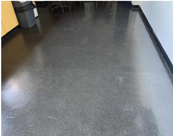
Line ID 37: Internal, Main Arena 1, Western Storage Area, F.03 Floor Covering, Black Vinyl Sheet - No Asbestos Detected
