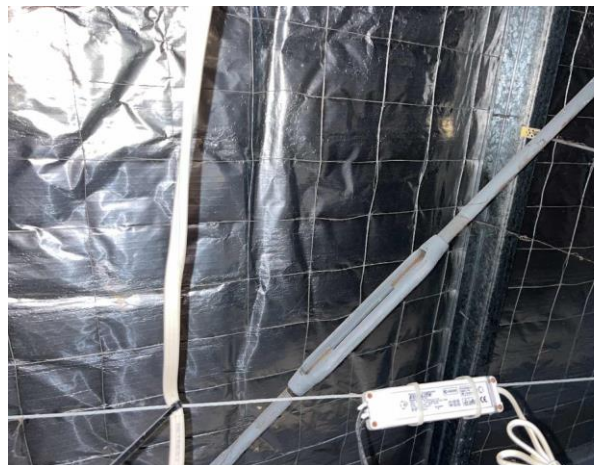
Line ID 78: Internal, Riders Retreat, Throughout, Ceiling Space, Sarking Insulation - Suspected SMF
