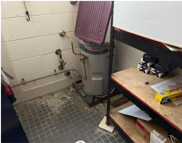
Line ID 75: Internal, Riders Retreat, Bathrooms, Cleaners Store, Hot Water Heater, Internal Insulation - Suspected SMF
