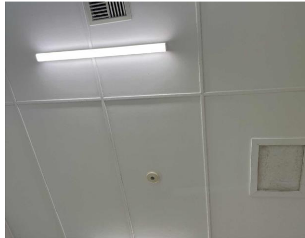
Line ID 25: Internal, House, Board Room, Ceiling, Fibre Cement Sheet - Chrysotile Asbestos Detected
