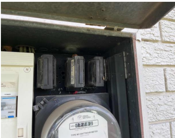
Line ID 16: External, House, Perimeter, Switchboard, HRC Fuses - Suspected Asbestos
