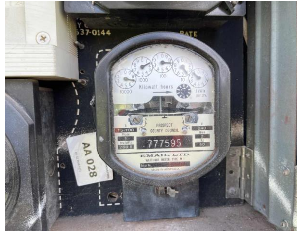
Line ID 14: External, House, Perimeter, Meter Box, Mastic Sealant to Meter - Suspected Asbestos
