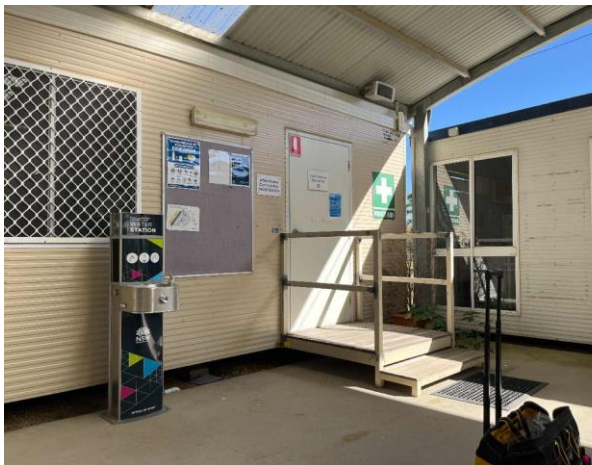
Line ID 66: External, Riders Retreat, First Aid Room, Walls and Handrails, Cream Paint - Lead Detected (<0.005% w/w)
