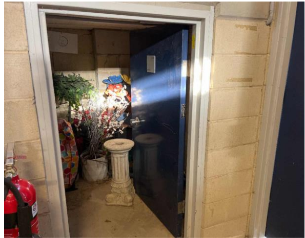
Line ID 32: Internal, Main Arena 1, Eastern Storage Area, Door to E.05, E.04 and E.03, Fire Door Core - Suspected Asbestos
