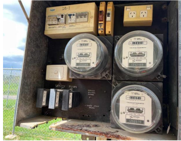
Line ID 2: External, Gardeners Shed, Electrical Box, Switchboard, HRC Fuses - Suspected Asbestos
