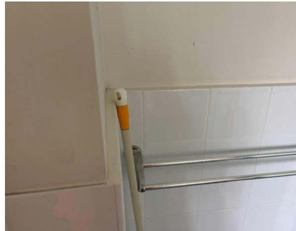
Line ID 24: Internal, House, Bathroom, Walls Behind Tiles, Fibre Cement Sheet - Suspected Asbestos
