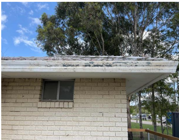
Line ID 63: External, House, Perimeter, Gutters, White Paint - Lead Detected (0.12% w/w)
