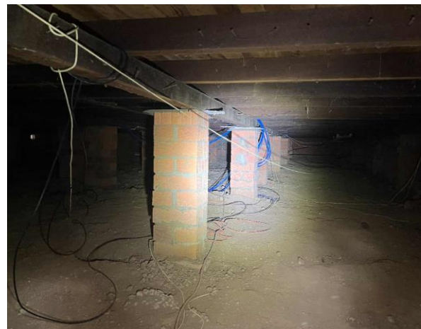
Line ID 28: Internal, House, Board Room, Sub Floor Packers, Fibre Cement Sheet - Suspected Asbestos
