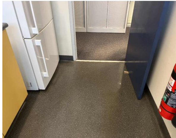
Line ID 54: Internal, Venue Office, Kitchen, Floor Covering, Grey Vinyl Sheet - No Asbestos Detected
