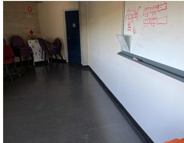
Line ID 38: Internal, Main Arena 1, Western Storage Area, F.03 Skirting, Black Vinyl Sheet - No Asbestos Detected
