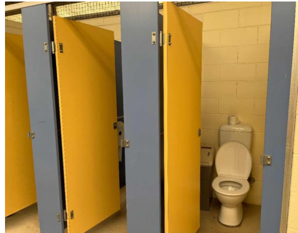
Line ID 42: Internal, Main Arena 1 West Amenities, Female Toilets, Partition Walls, Fibre Cement Sheet - No Asbestos Detected
