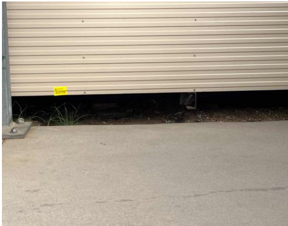
Line ID 19: External, Riders Retreat, First Aid Room, Packers Under Floor, Fibre Cement Sheet - No Asbestos Detected
