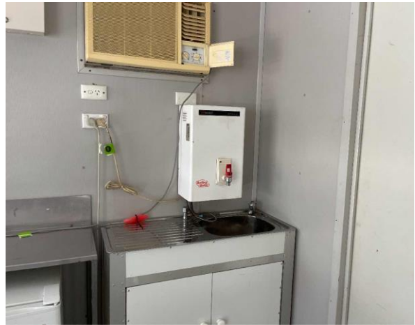
Line ID 76: Internal, Riders Retreat, Event Office, Above Sink, Hot Water Boiler, Internal Insulation - Suspected SMF
