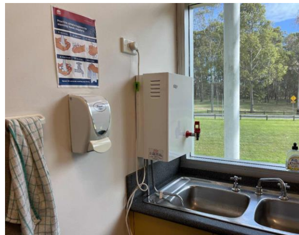
Line ID 84: Internal, Venue Office, Kitchen, Above Sink, Boiler, Internal Insulation - Suspected SMF
