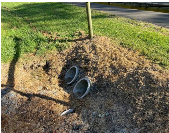
Line ID 4: External, Grounds Throughout, North Side of Cabins, Drainage Pipes, Moulded Fibre Cement - No Asbestos Detected
