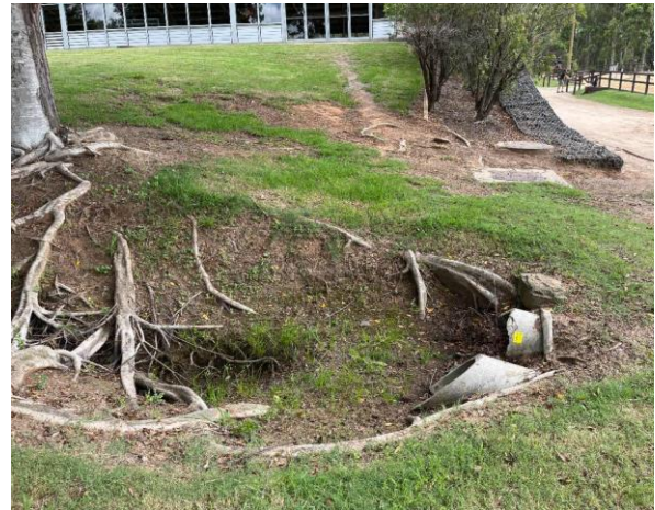
Line ID 6.1: External, Grounds Throughout, South of Indoor Arena, Drainage Pipes, Moulded Fibre Cement - No Asbestos Detected
