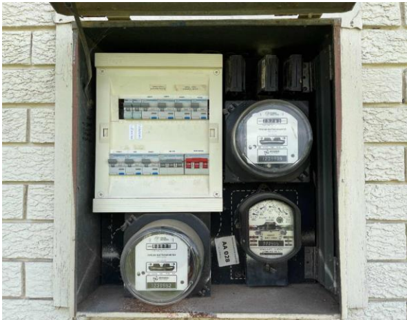
Line ID 13: External, House, Perimeter, Meter Box, Bituminous Backing Board - Suspected Asbestos
