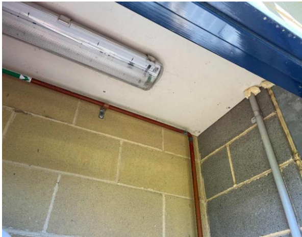
Line ID 43: Internal, Northern Amenities, Store Room, Ceiling, Fibre Cement Sheet - No Asbestos Detected
