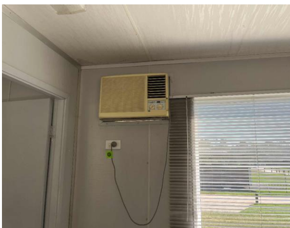
Line ID 92: Internal, Riders Retreat, Event Office, TECO AC Unit, Unknown Refrigerant - Suspected ODS
