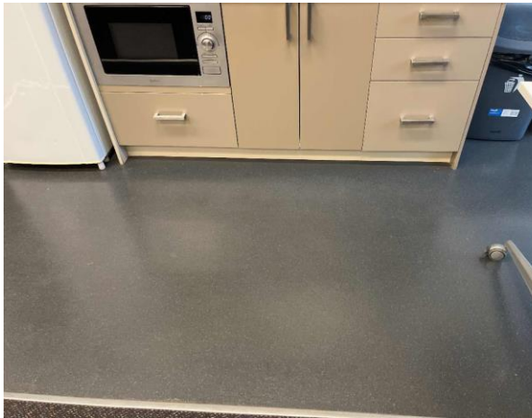
Line ID 53: Internal, Venue Office, Conference Room, Kitchen Area, Floor Covering, Grey Vinyl Sheet - No Asbestos Detected
