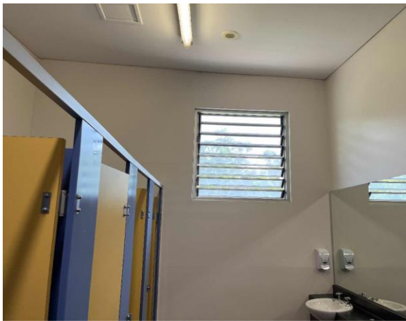
Line ID 60: Internal, Venue Office, Toilets, Walls, Fibre Cement Sheeting - No Asbestos Detected
