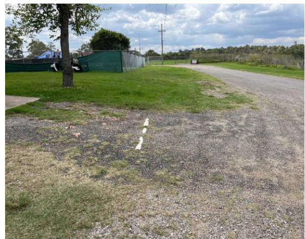
Line ID 10: External, House, Front of House, Driveway, Pipework, Fibre Cement Sheet - Chrysotile, Amosite and Crocidolite Asbestos Detected
