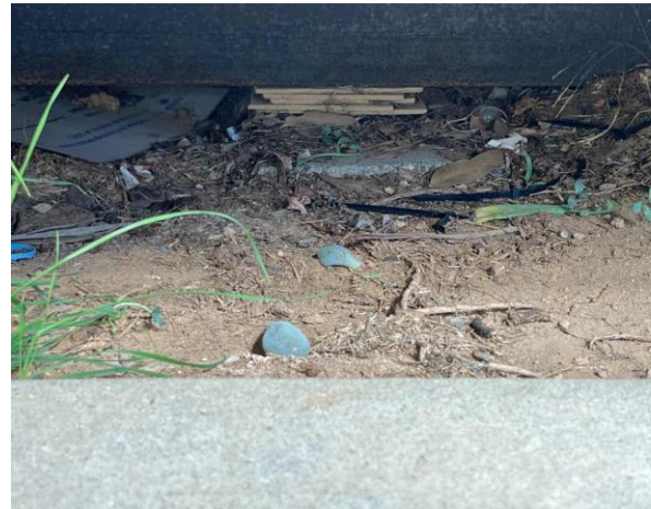
Line ID 19.1: External, Riders Retreat, First Aid Room, Packers Under Floor, Fibre Cement Sheet - No Asbestos Detected
