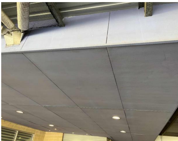
Line ID 20: External, Venue Office, Throughout, Fascia and Ceiling, Fibre Cement Sheet - No Asbestos Detected
