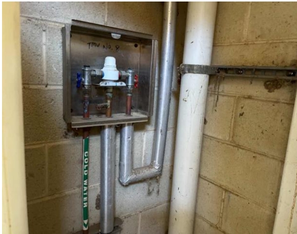
Line ID 80: Internal, Stables, Amenities, HWS Cupboards, Pipework, Insulation Material - Suspected SMF
