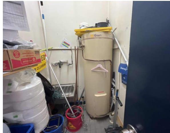
Line ID 81: Internal, Venue Office, Cleaners Store A.10, Hot Water Heater, Internal Insulation - Suspected SMF
