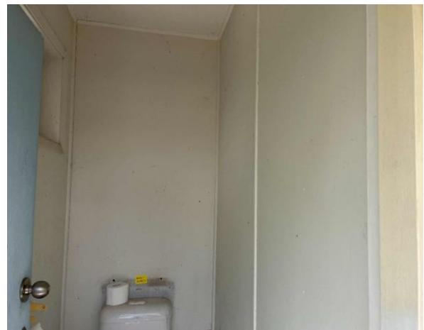
Line ID 17: External, House, Perimeter, Toilets, Walls and Ceilings, Fibre Cement Sheet - Chrysotile Asbestos Detected
