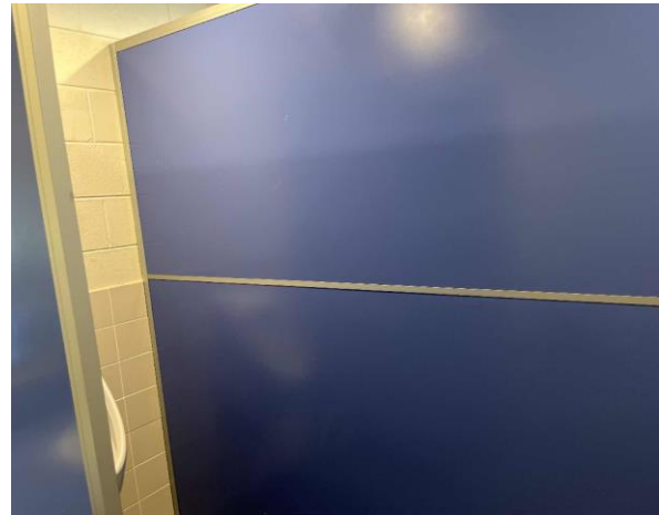
Line ID 44: Internal, Riders Retreat, Bathrooms, Cubicle Partition Walls, Fibre Cement Sheet - No Asbestos Detected
