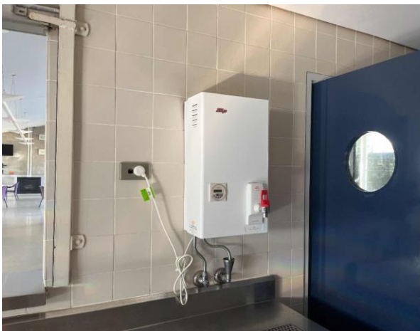
Line ID 77: Internal, Riders Retreat, Kitchen, Hot Water Boiler, Internal Insulation - Suspected SMF
