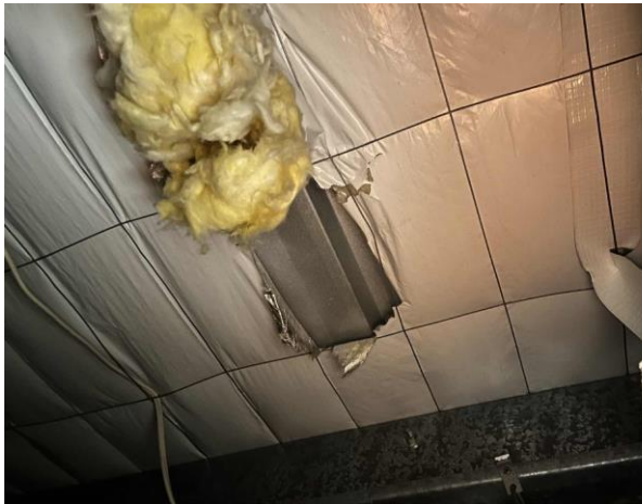
Line ID 87: Internal, Venue Office, Throughout, Ceiling Space, Sarking Insulation - Suspected SMF
