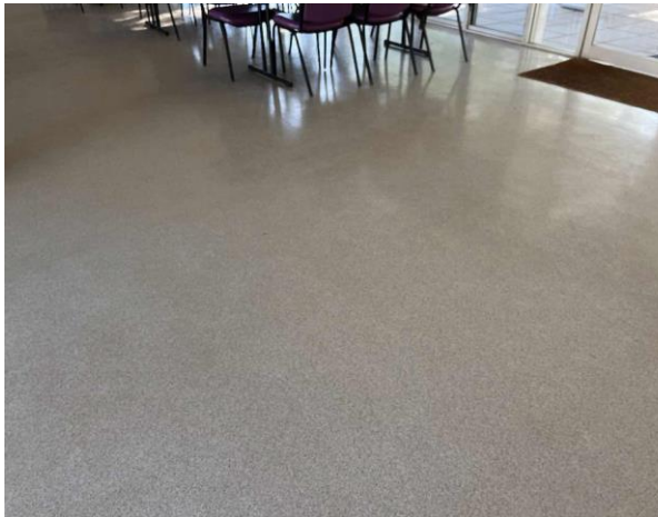
Line ID 47: Internal, Riders Retreat, Throughout, Floor Covering, Blue Vinyl Sheet - No Asbestos Detected
