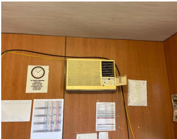
Line ID 95: Internal, Security Office, Throughout, TECO AC Unit, Unknown Refrigerant - Suspected ODS
