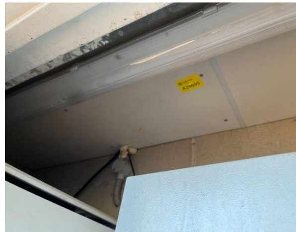
Line ID 40: Internal, Main Arena 1 West Amenities, C.08 Store, Ceiling, Fibre Cement Sheetting - No Asbestos Detected
