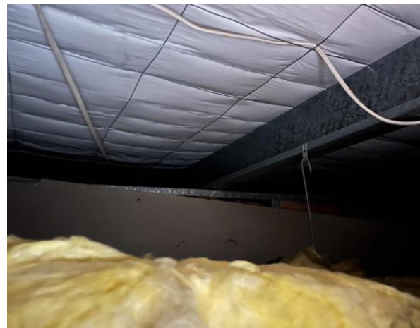
Line ID 86: Internal, Venue Office, Throughout, Ceiling, Insulation Batts - Suspected SMF
