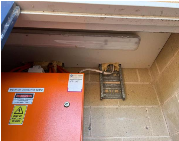
Line ID 41: Internal, Main Arena 1 West Amenities, C.09 Distribution Board, Ceiling, Fibre Cement Sheeting - No Asbestos Detected
