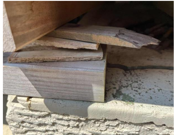
Line ID 8: External, House, Backyard, Packers Under Deck, Fibre Cement Sheet - No Asbestos Detected
