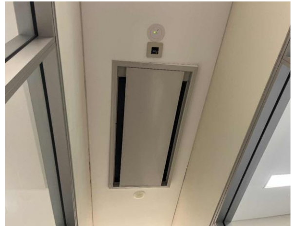
Line ID 88: Internal, Venue Office, Throughout, Ceiling Space, Air Conditioning Ductwork - Suspected SMF
