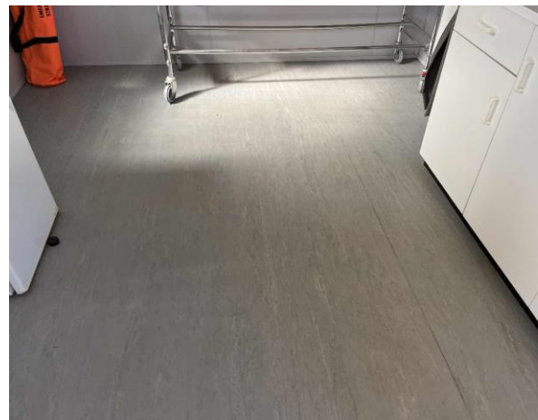
Line ID 46: Internal, Riders Retreat, First Aid Room, Floor Covering, Blue Vinyl Sheet - No Asbestos Detected
