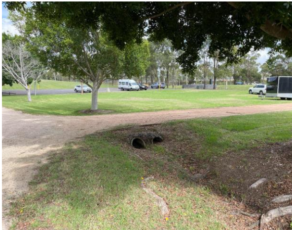
Line ID 6: External, Grounds Throughout, South of Indoor Arena, Drainage Pipes, Moulded Fibre Cement - No Asbestos Detected
