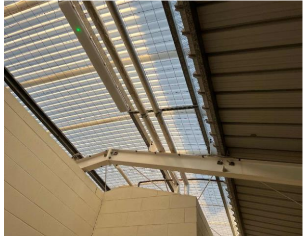
Line ID 74: Internal, Main Arena 1 West Amenities, Female Toilets, Pipework, Insulation Material - Suspected SMF
