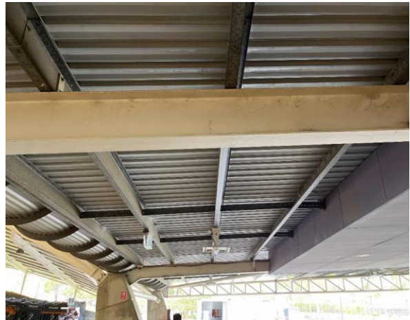
Line ID 65: External, Indoor Arena, Throughout, Beams, White Paint - Lead Detected (<0.005% w/w)
