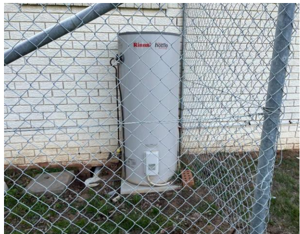
Line ID 70: External, House, Perimeter, Hot Water Heater, Insulation Material - Suspected SMF
