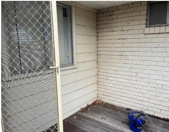
Line ID 18: External, House, Perimeter, Walls, Weatherboard Cladding, Fibre Cement Sheet - No Asbestos Detected
