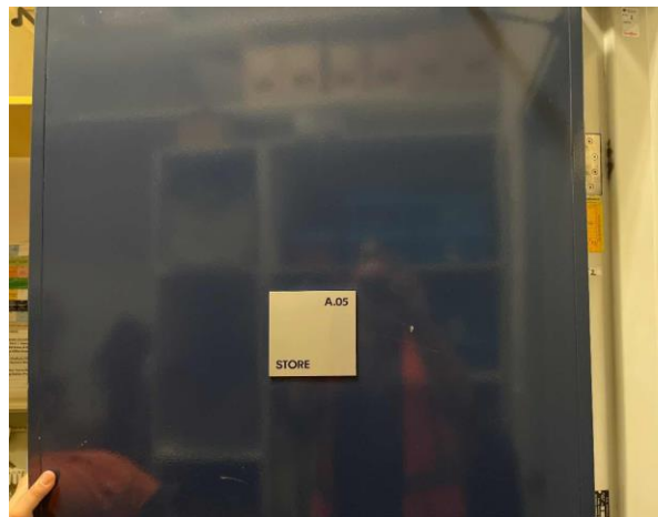
Line ID 56: Internal, Venue Office, Office A.05, Fire Door, Fire Door Core - Suspected Asbestos
