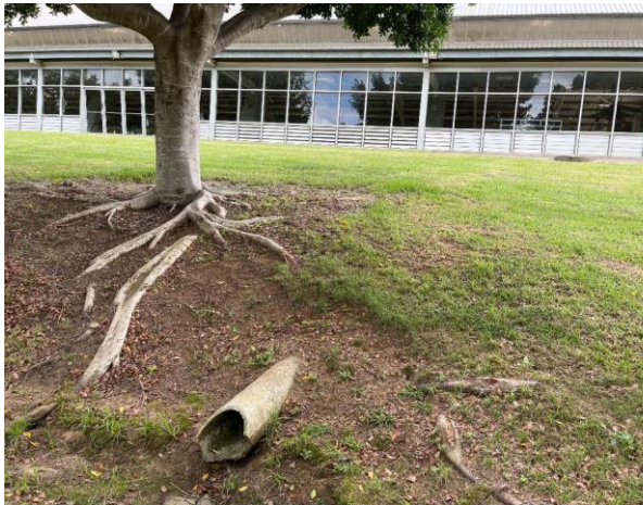
Line ID 7: External, Grounds Throughout, South of Indoor Arena, Smaller Drainage Pipe, Fibre Cement Sheet - No Asbestos Detected
