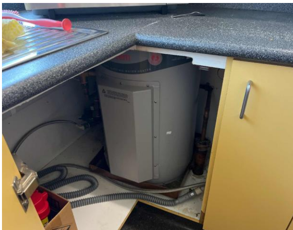
Line ID 85: Internal, Venue Office, Kitchen, Hot Water Heater, Internal Insulation - Suspected SMF
