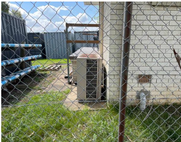
Line ID 90: External, House, Backyard, AC Unit, Unknown Refrigerant - Suspected ODS
