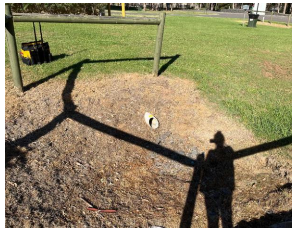
Line ID 5: External, Grounds Throughout, North Side of Cabins, Small Drainage Pipes, Compressed Cement Sheet - No Asbestos Detected
