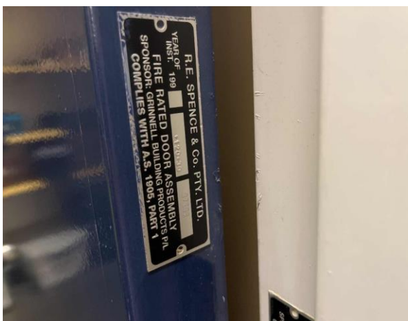
Line ID 56.1: Internal, Venue Office, Office A.05, Fire Door, Fire Door Core - Suspected Asbestos
