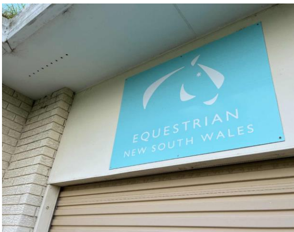
Line ID 9: External, House, Front of House, Above Garage Door, Infill Panel, Fibre Cement Sheet - No Asbestos Detected
