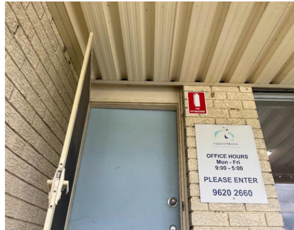
Line ID 18.1: External, House, Perimeter, Walls, Weatherboard Cladding, Fibre Cement Sheet - No Asbestos Detected
