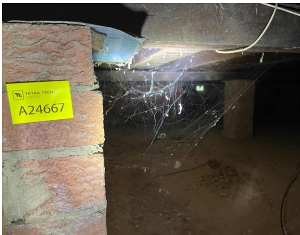
Line ID 27: Internal, House, Board Room, Sub Floor, Bituminous Packers - No Asbestos Detected
