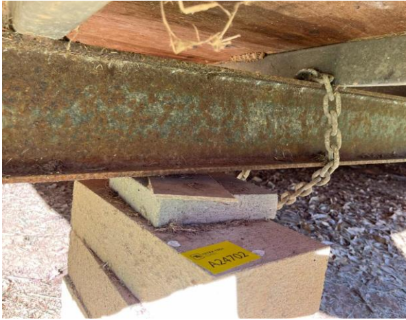
Line ID 1: External, Cabins, Throughout, Packers Under House, Fibre Cement Sheet - No Asbestos Detected
